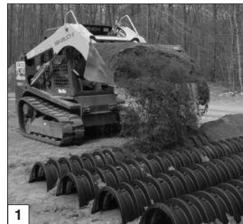
Ladle soil on chamber domes.
